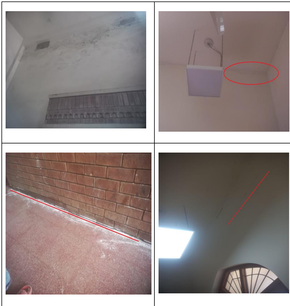
Visible Cracks in walls and floor of the Railway Station building, Raiwind
